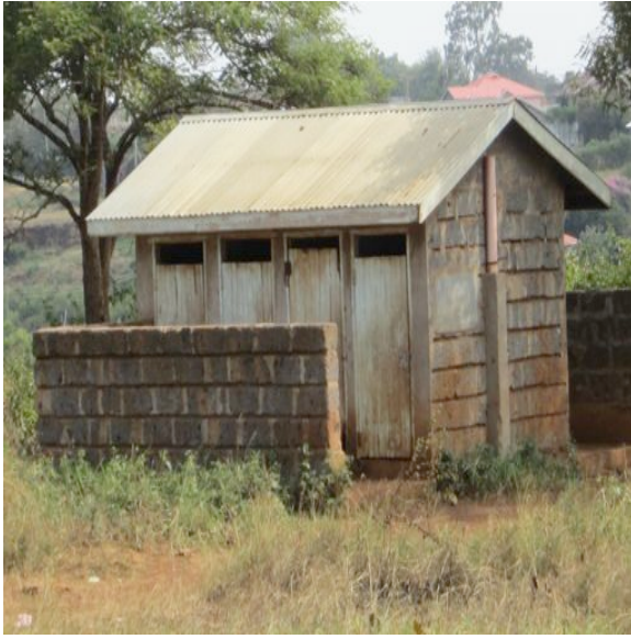
State of girl's latrine before renovation
