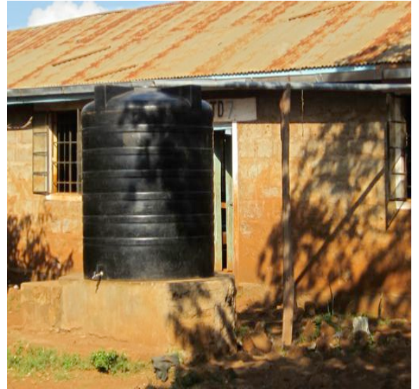
complete rain water harvesting system
