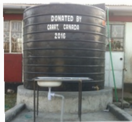
WATER CATCHMENT SYSTEM AND HAND-WASHING STATION AT THE HOPE SCHOOL, MBITA, KENYA
